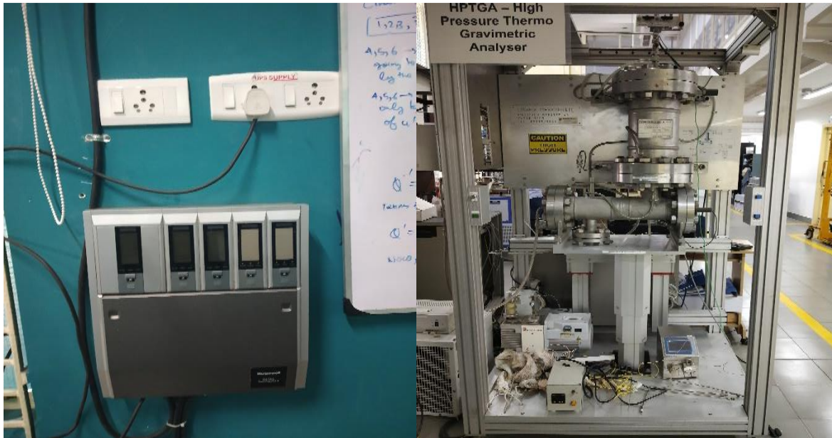
GAS Detector for Hydrogen gas
