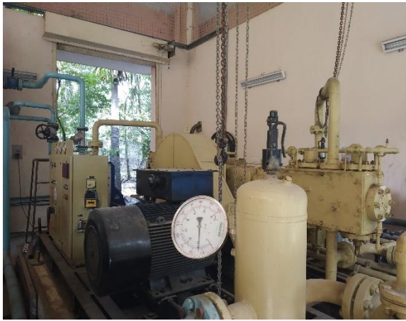
Reciprocating compressor- 2stage 120hp Supply of air at 40 bar
