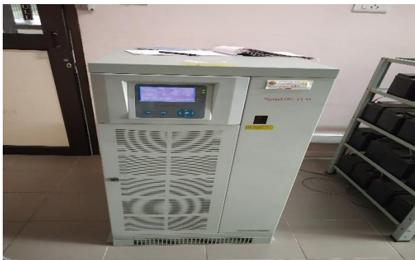
UPS system with power-10kva
