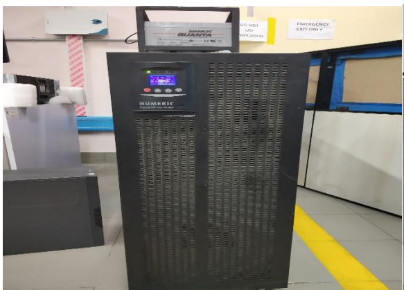
UPS system with dc power pack 10kva
