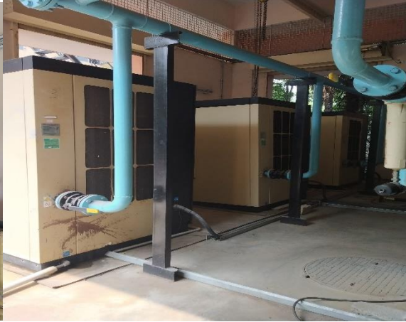
Ingersoll rand screw Air compressor-3no to supply at 10 bar
