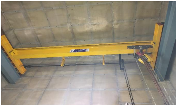
Hand operated overhead travelling Crane
